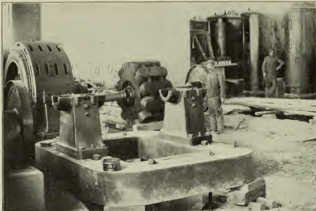
INTERIOR OF THE POWER STATION AND TRANSFORMER ROOM DURING CONSTRUCTION. kilowatts capacity, placed in oil and cooled with water circulation provided by two small motor pumps run by the exciting machines. The transformers raise the pressure from 3,000 to 30,000 volts, and at
